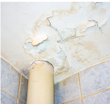
Damp through penetration/ rupture
