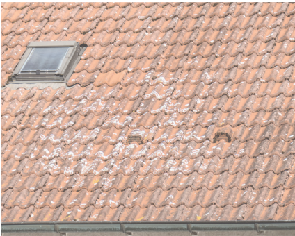
Damp through penetration/roof
