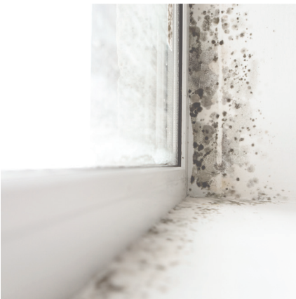
Condensation damp. Mould
