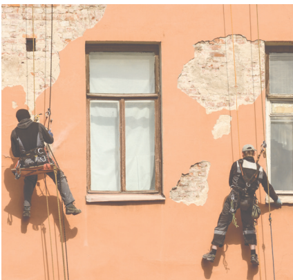
Damp through penetration/ façade
